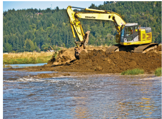
Skokomish River delta restoration work photo by Paul Cereghino, NOAA Restoration Center.
